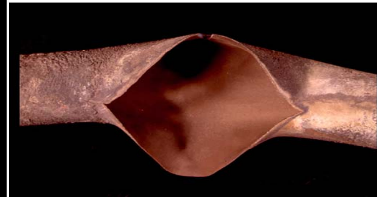
Fishmouth' High-Temperature Failure Of Waterwall Tube
